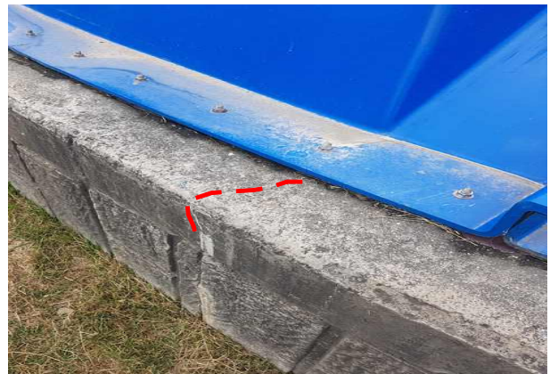
벽체 균열 (CW=0.2mm, L=1.0m, 4EA)
